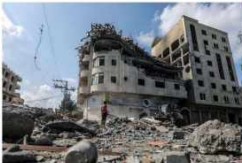
A destroyed Paltel building in Gaza City in October. Credit: Mohammed Saber/EPA, via Shutterstock
